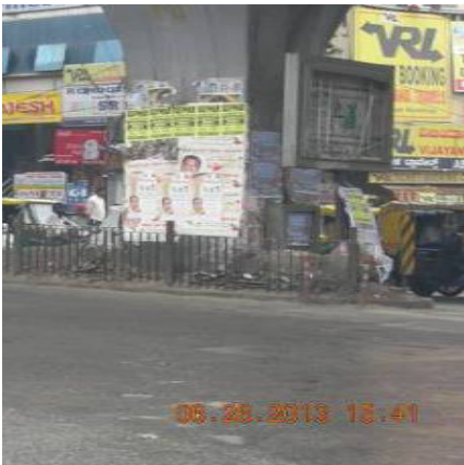
Damaged advertisement boards and posters pasted on the landscape of the Anandrao Circle flyover
