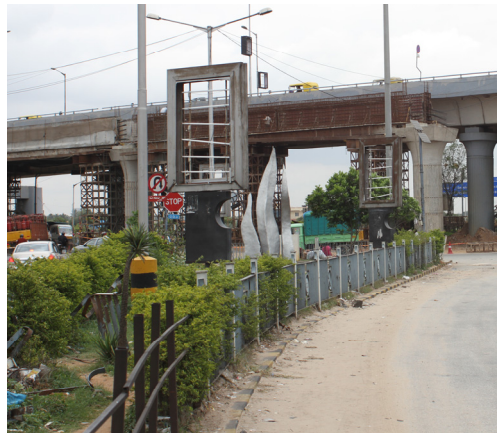
Damaged advertisement boards at Hebbal flyover
