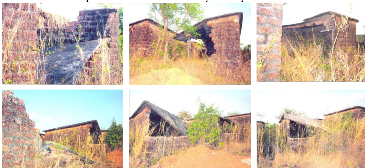
(Collapsed roofs and walls of Ashraya houses)
